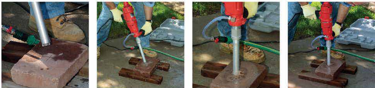
Determine location of hole; Turn on water at valve, hold at 45° angle start drill and set on paver; As drill bit gets started, straighten to 90°; add pressure and drill through paver.
